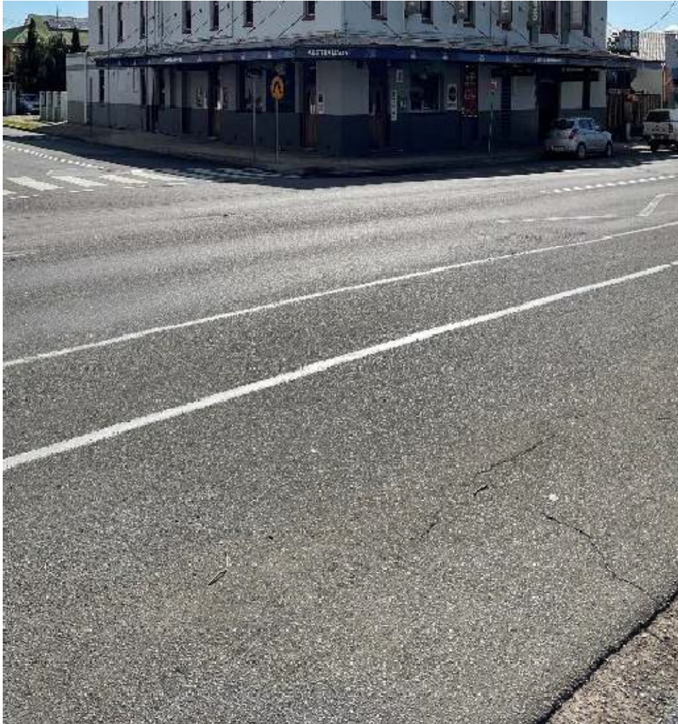
Figure 6 The road surface and kerbside guttering in front of the Australia Hotel in Cessnock
