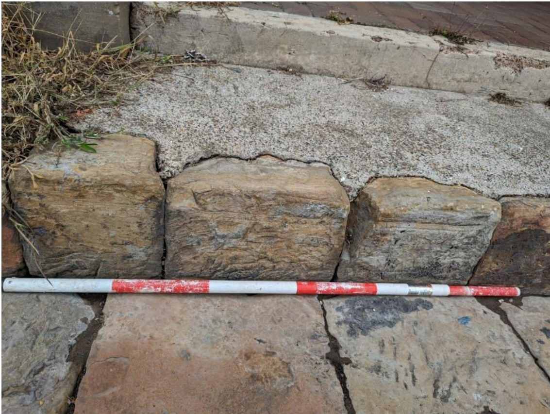
Figure 6. Sandstone kerb in front of the Bellbird Hotel with signs of potential pick marks on upper blocks, drill marks on the third and second blocks on front faces and evidence of more recent concreting.
