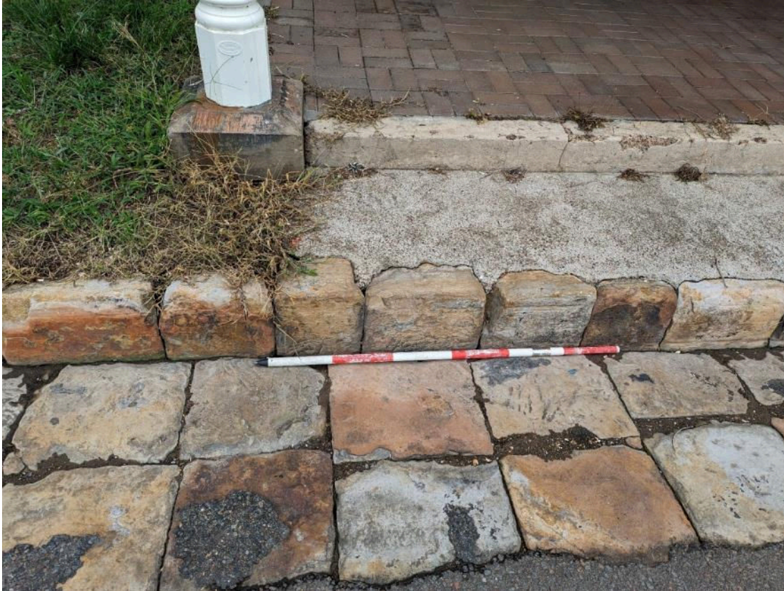
Figure 7. Sandstone kerb and guttering in front of the Bellbird Hotel showing impacts of tarring and cementing.
