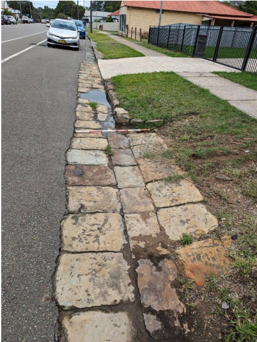
Figure 8. Sandstone kerb in the project area with sandstone driveway and cut-in cement driveway.
