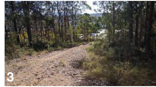
3 Millfield Street road reservation. Unformed, eroding.
